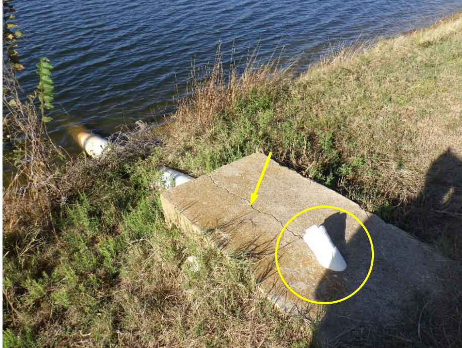
Photo 17. View of the siphon pipe and concrete anchor block with air inlet plug (circled) near mid dam on the upstream slope. Note the crack (arrow) on the anchor block is still present as observed in previous inspections.
