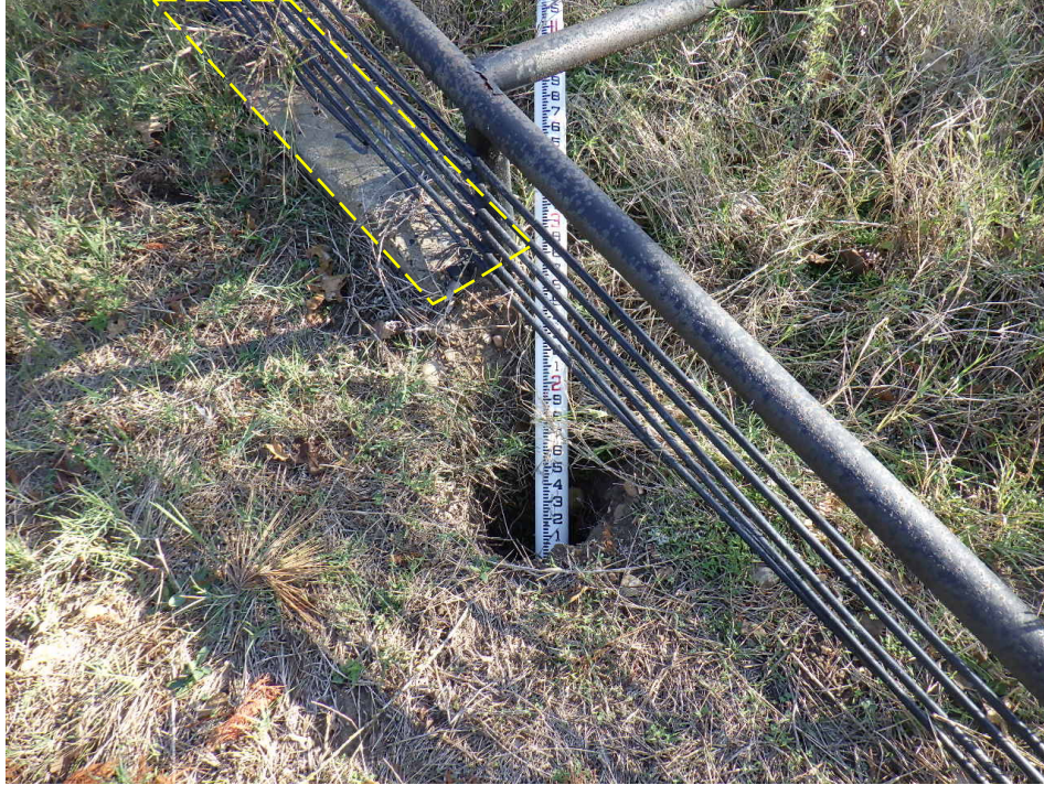
Photo 15. View of burrow/hole along the debris guard fence and near the right end of the concrete weir (dashed line). Note the burrow/hole measured approximately 1.4-feet deep.
