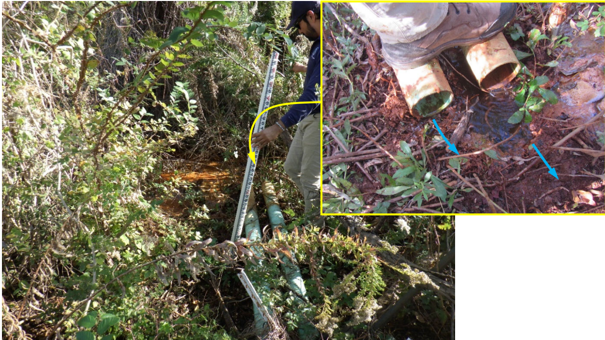
Photo 13. View of the two 4-inch PVC drainpipes within the overgrown downstream area. Note the pipes were angled slightly upwards; therefore, creating negative drainage and not properly draining.
