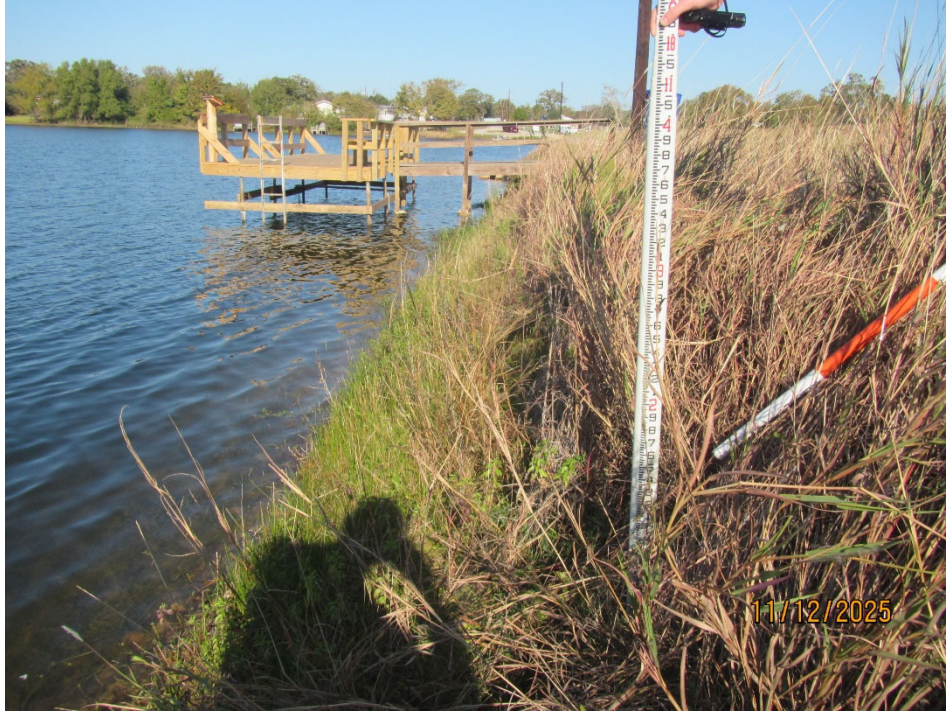
Photo 7. View of benching occurring near the right end the upstream slope looking left. Note the taller grass growth obstructing the approximate 1.5-foot high bench along the approximate normal pool elevation.
