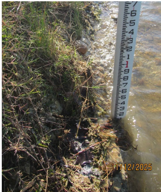
Photo 6. View of minor benching occurring along the mid-left end of the upstream slope along the shoreline. Benching in this area measured approximately 1-foot high.
