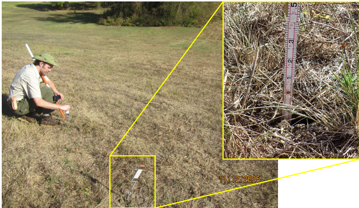
Photo 11. View of an area along the lower downstream slope at the right end of the dam where several longitudinal cracks were observed. Note the most significant crack measured approximately 11-inches deep.
