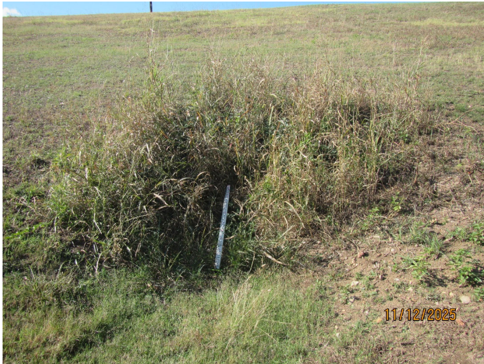
Photo 10. View of an area believed to be the location of the siphon pipe outlet but noted in the previous report to be a new slide. Note the outlet was not observed and the area was overgrown with grass.
