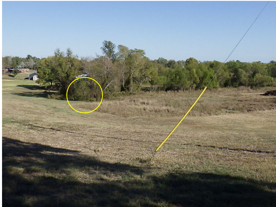
Photo 12. View of the dense vegetative growth along the downstream toe area where the two 4-inch PVC pipes (circled) discharge.
