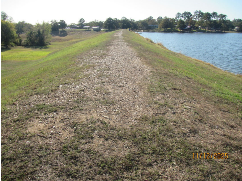
Photo 3. View of the crest looking right from the mid-left end of the dam. Note the bare soil area along the crest.
